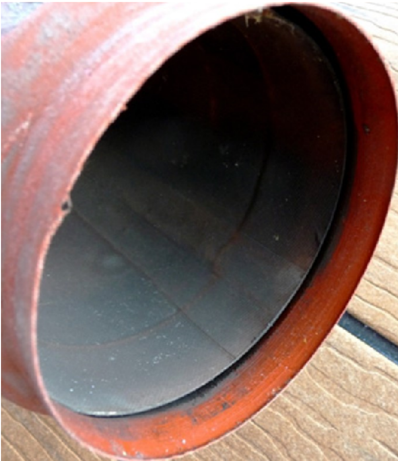
Contaminated Air Duct. Quelle: AERO
